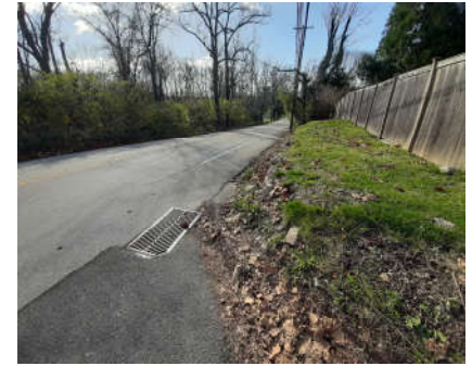
Roadside obstructions near Township Line Road, Whitpain Township
