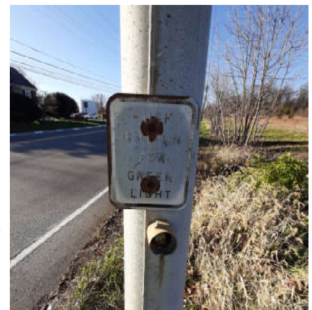
Inoperable Pedestrian Signal Equipment at the intersection of Germantown Pike with Trooper Road
