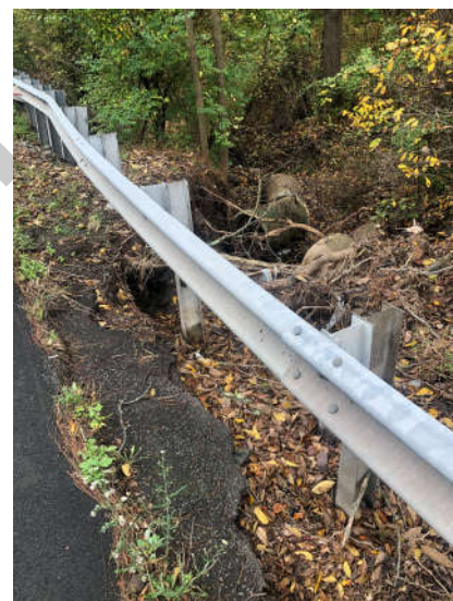
Erosion and deterioration of roadway pavement near Sankey Road intersection
